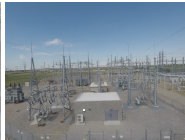
Overview of the substation. The north side that was rebuilt is on the right. The new control room is in the center of the picture.
