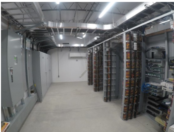
This is the back side of the relay panel in the new control room. It shows all of the wires and the connections that were made to get the substation up and operating.
