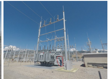
The newly installed transformer. If you look closely you can see the small-in-comparison sized BCLP employee standing next to the transformer.
