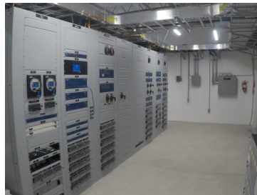
This is the front side of the relays that were installed in the new control room.
