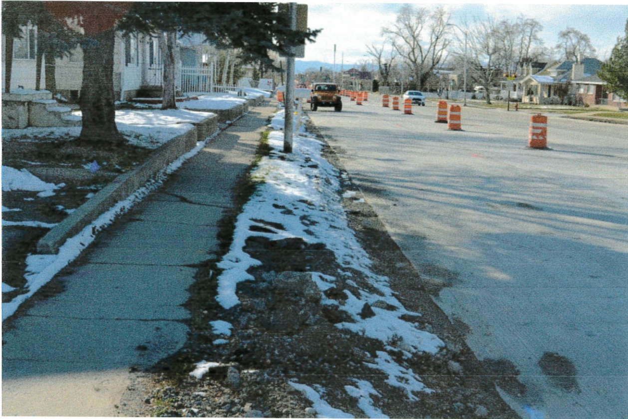
Steep slope sidewalk to curb.
