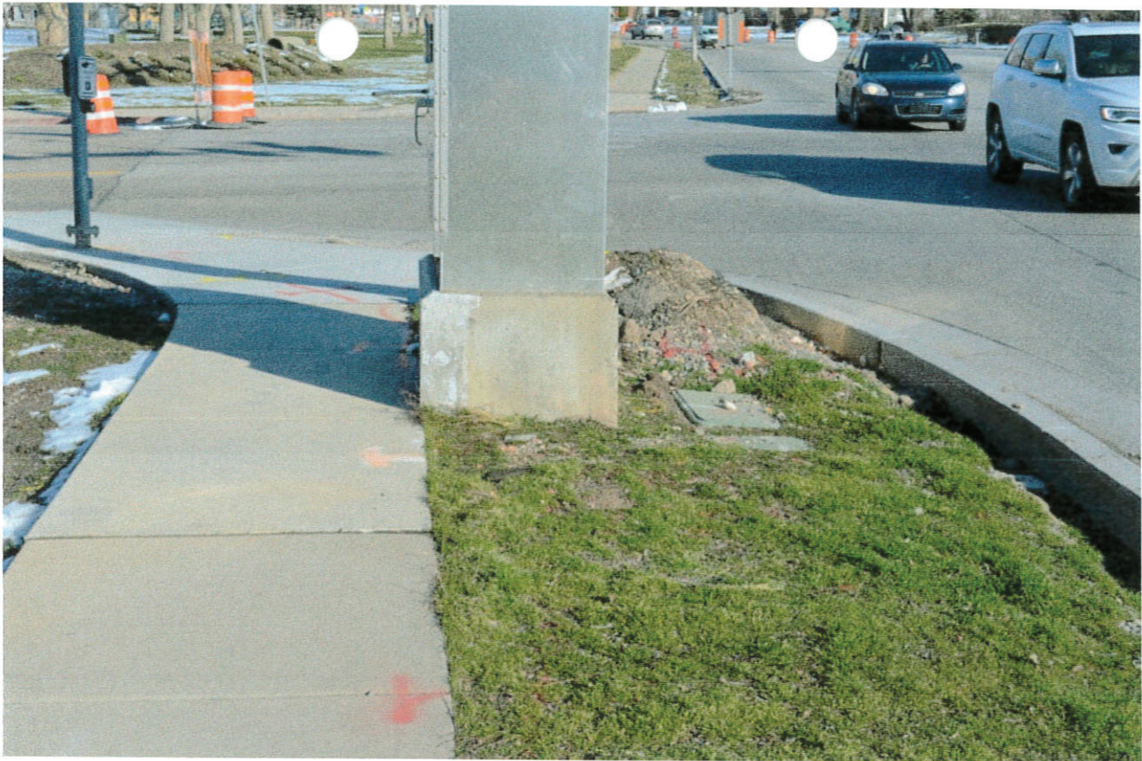
Utility crews pull onto park strip and damage sprinkler system. Owner desires hardscape to give them something to park on. Tired of Sprinkler repair.
