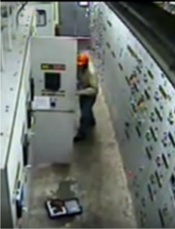
Photo of breaker cabinet before arc flash
