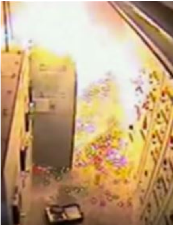
Photo of breaker during arc flash
