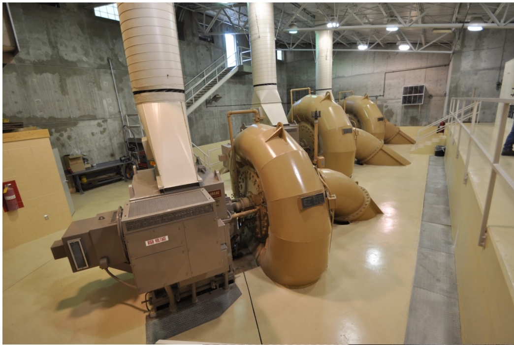
Overall picture of plant
