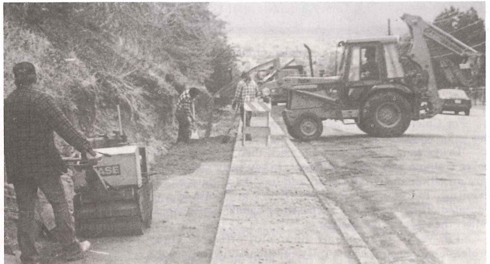
The 1800 South project will result in beautification and safety through a needed sidewalk and natural keystone retaining wall.
