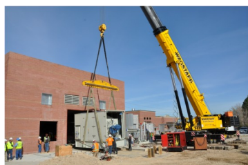
Delivery of one of the two generator sections of the new turbines at the BCLP plant on Tuesday, March 28, 2012
