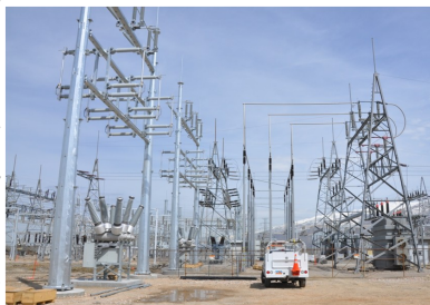
The substation can be seen from Legacy Highway at Parrish Lane in Centerville.
