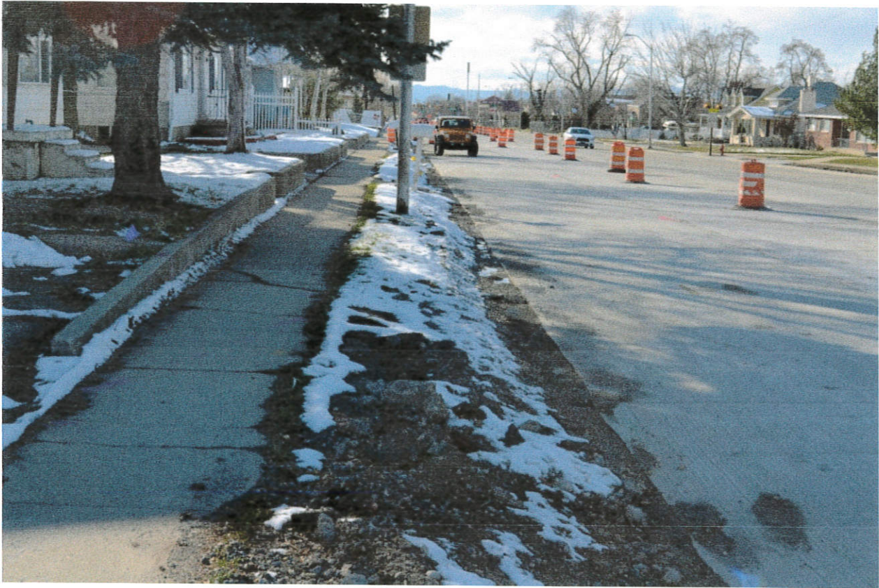
Steep slope sidewalk to curb.
