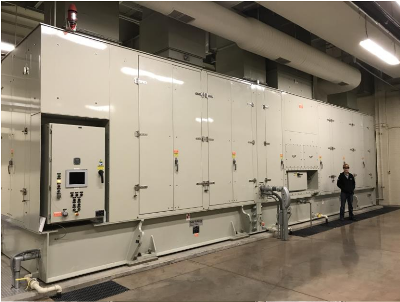
Entire Titan Turbine Package
