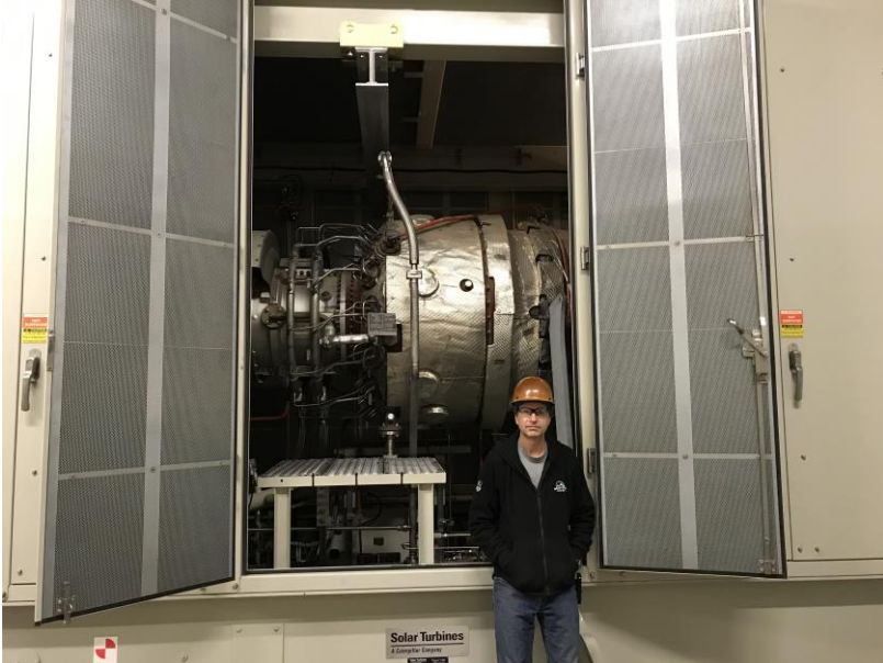
Titan motor inside enclosure
