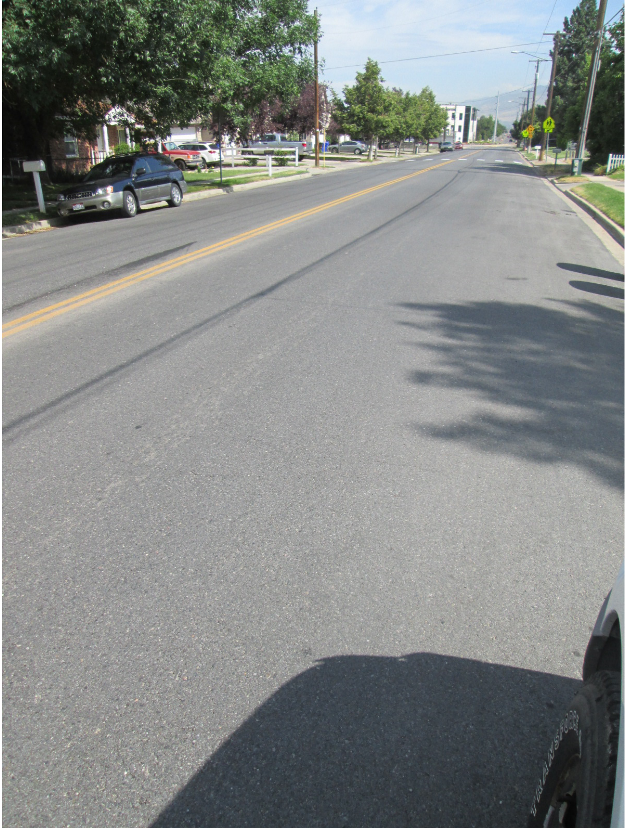
Photo 3. Good Condition – 200 W from 1700 S to 1500 S (RSL = 10 years)
