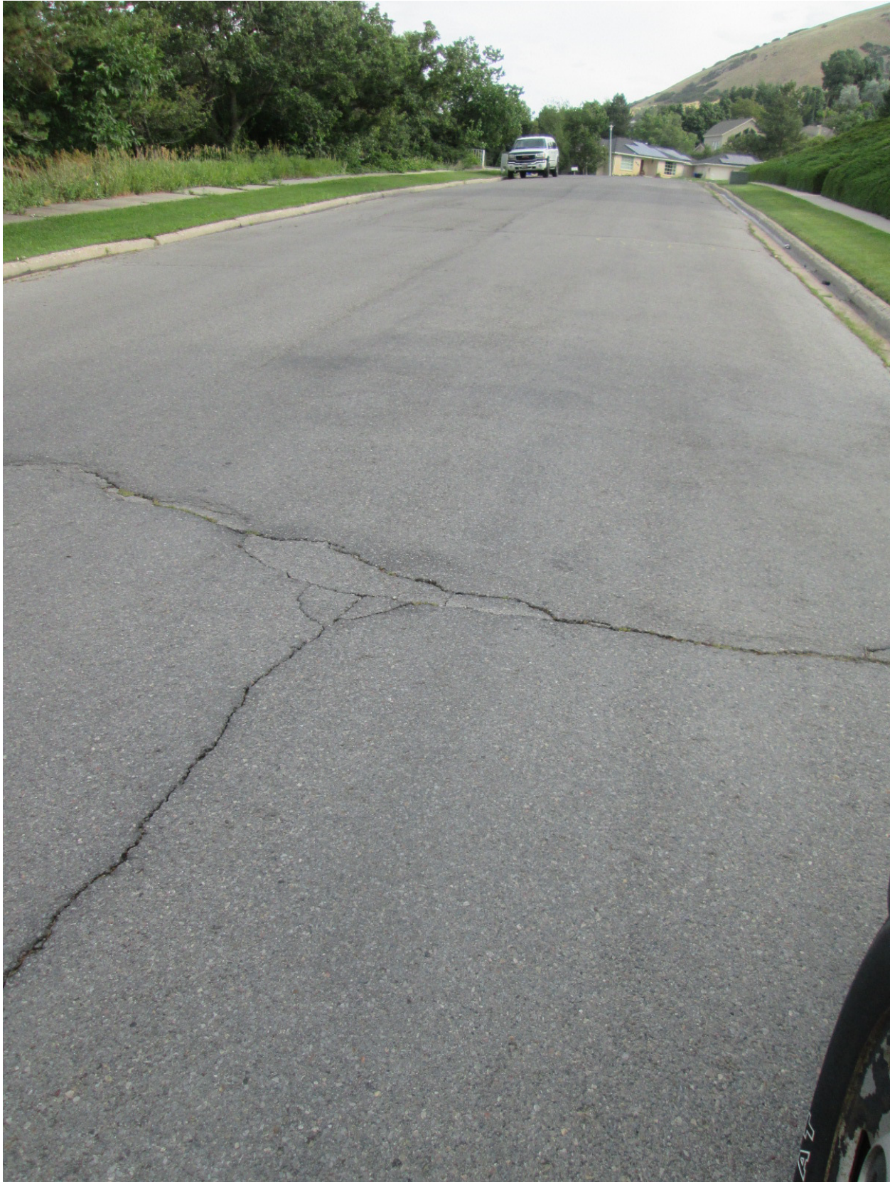
Photo 2. Fair Condition – 1200 E from 500 N to 700 N (RSL = 8 years)
