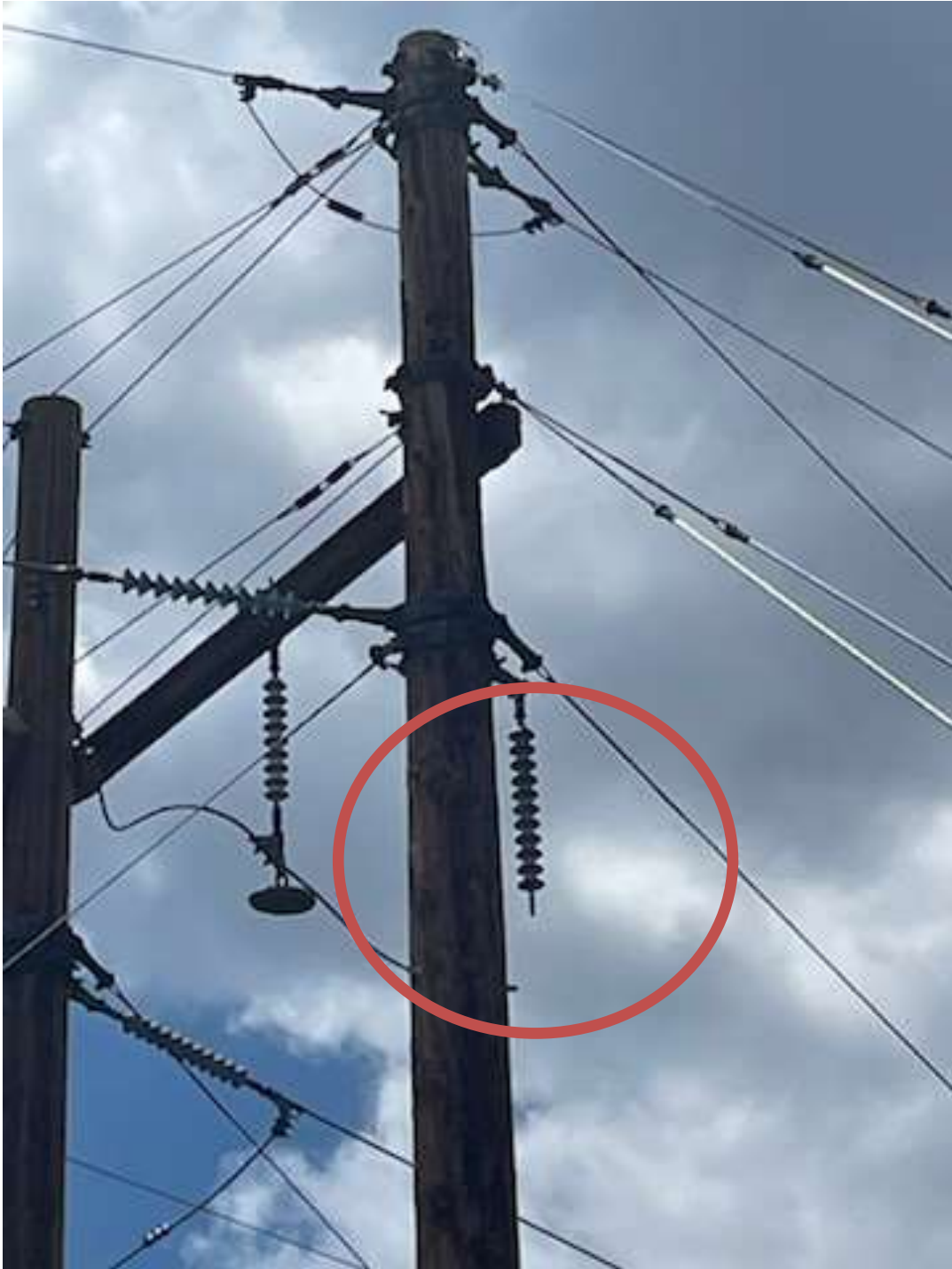
Failed Suspension Insulator
