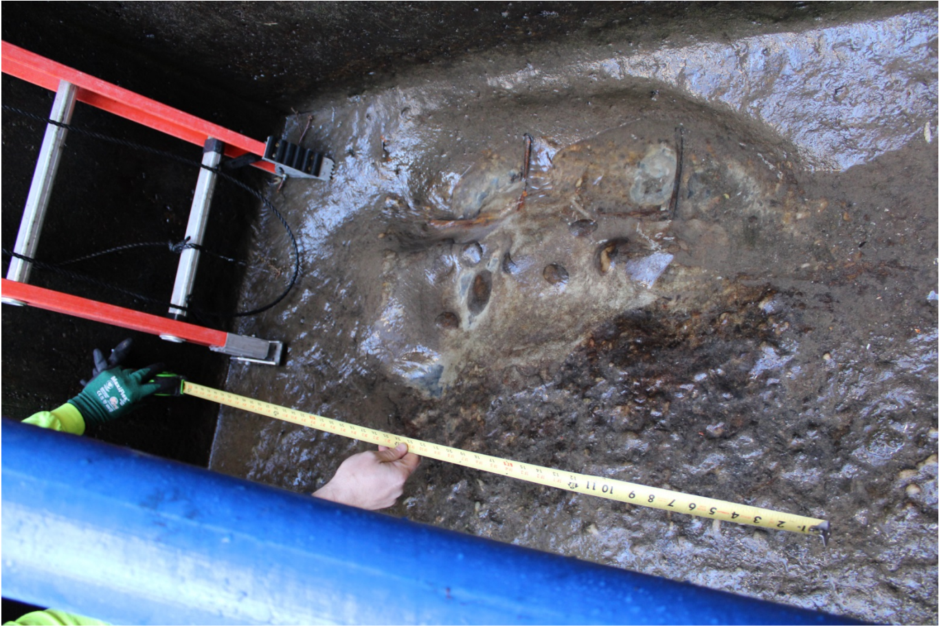
CONCRETE DAMAGE IN BAY 1 SHOWING EXPOSED REBAR
