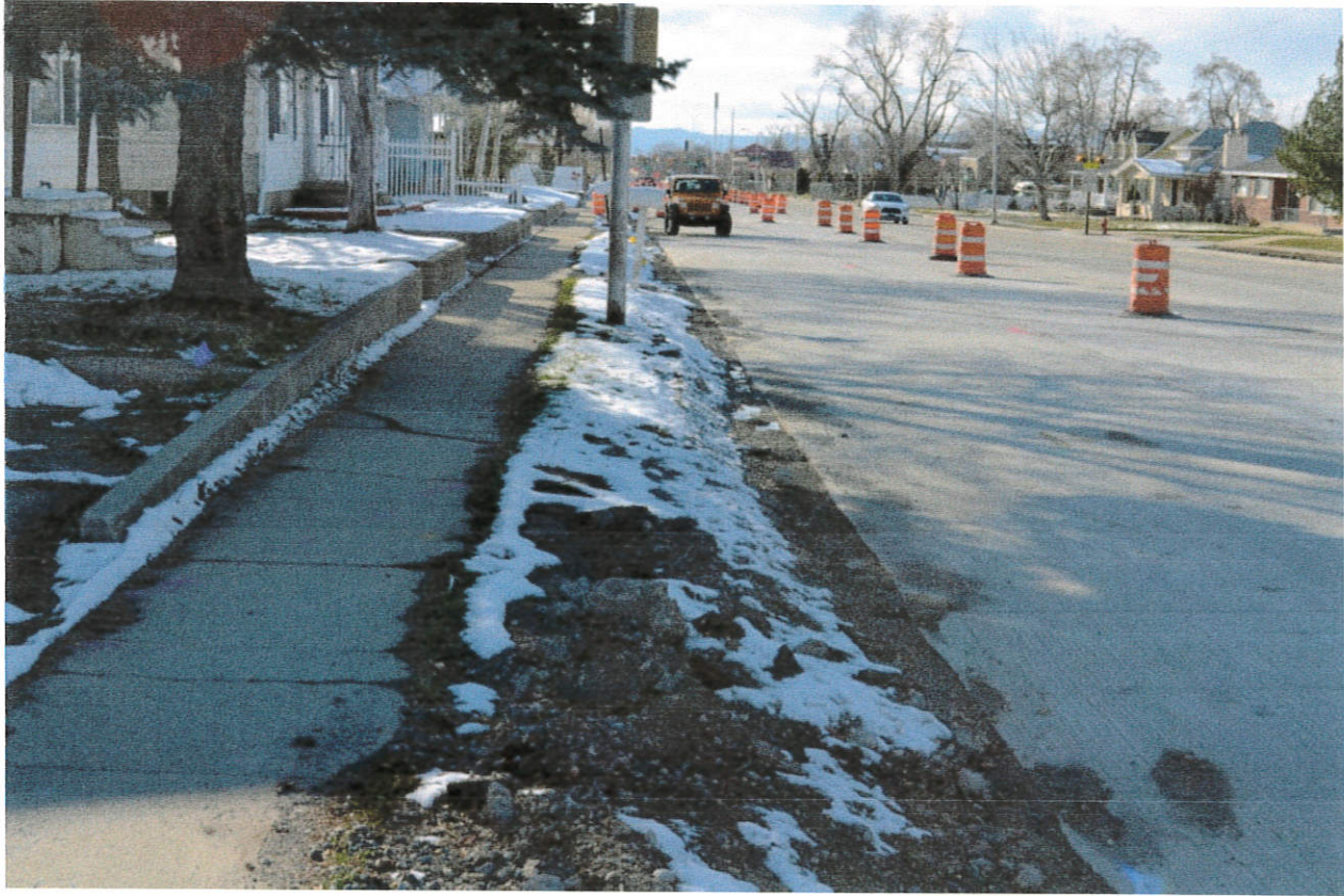
Steep slope sidewalk to curb.
