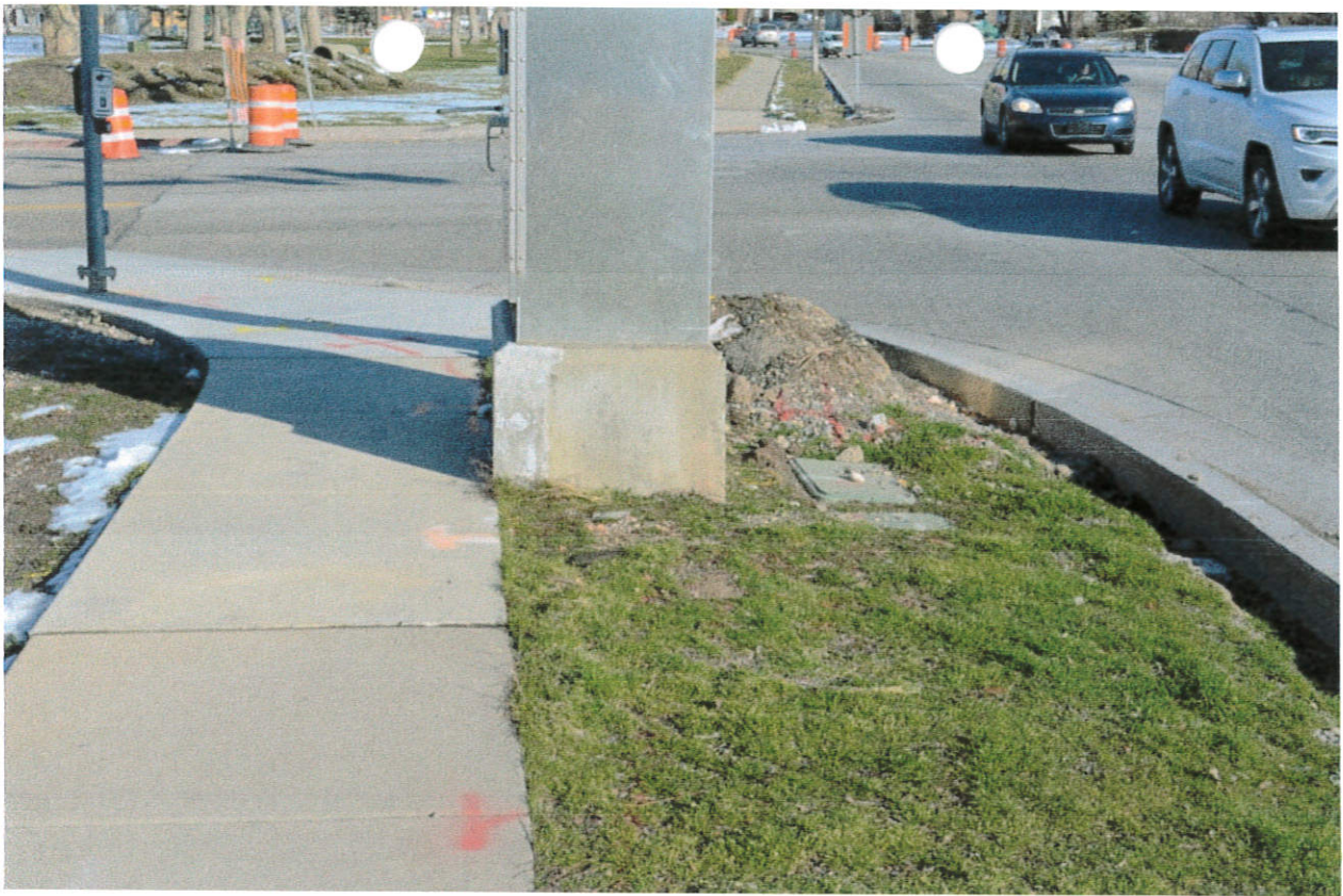
Utility crews pull onto park strip and damage sprinkler system. Owner desires hardscape to give them something to park on. Tired of Sprinkler repair.
