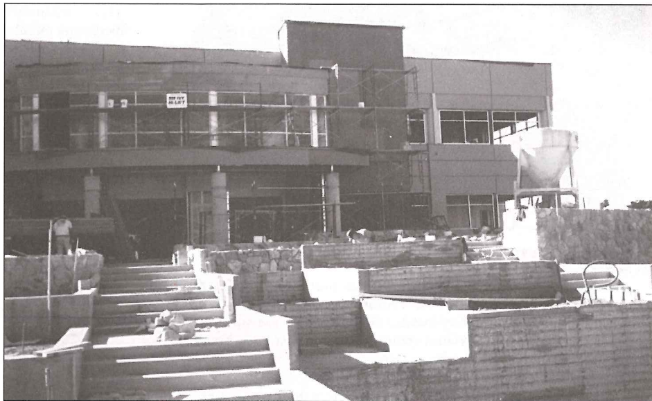
Chief Paul Rapp says the Public Safety Complex is a model of cost-effective planning and construction.
