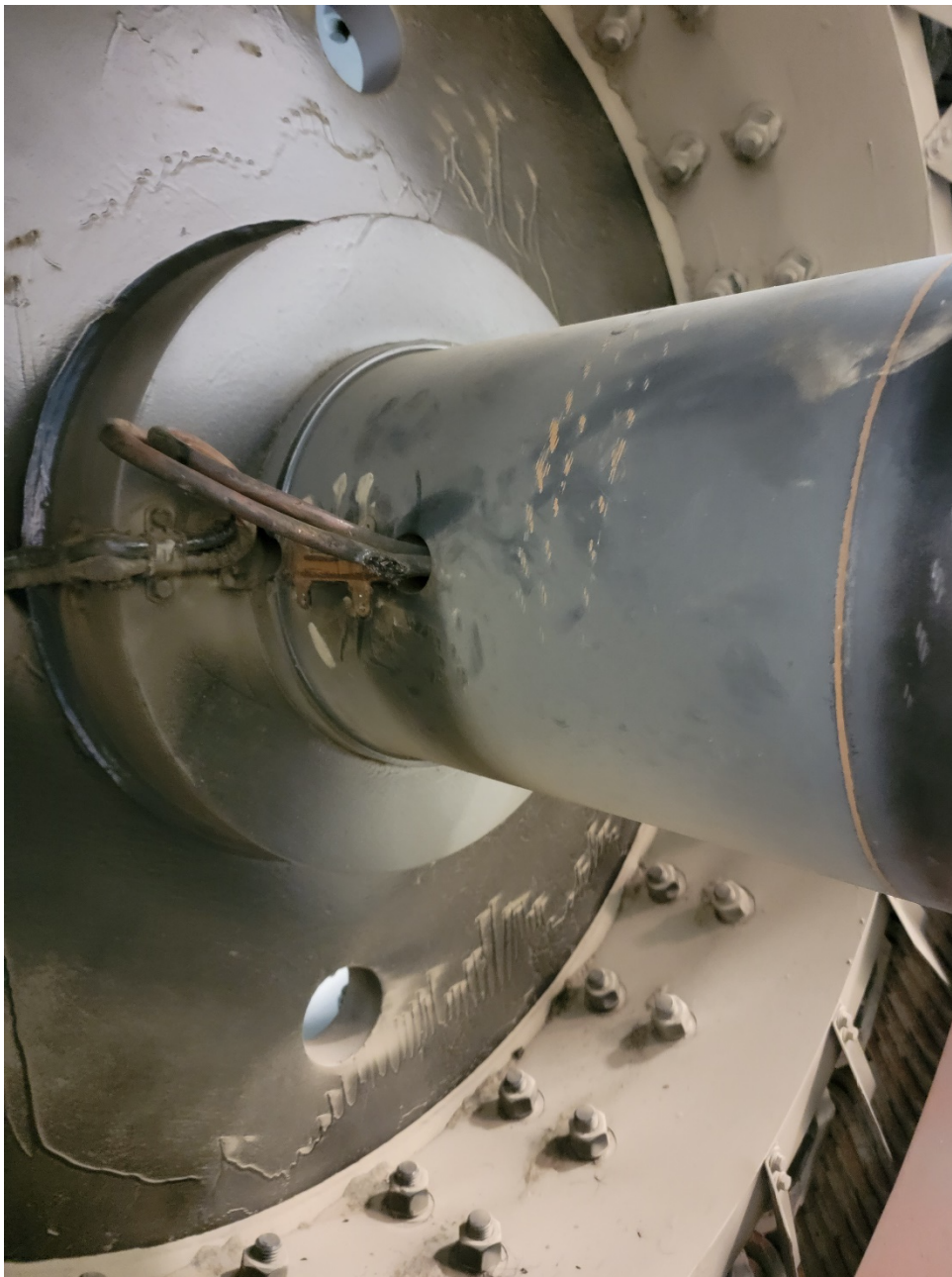
Shorted wire (the wire has been pulled out from the center of the rotor shaft)
